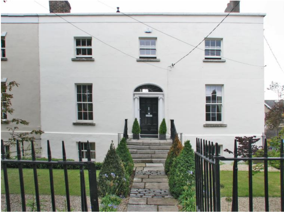
Mount Merrion Road, Blackrock Replacement of sash windows and landscaping to front
